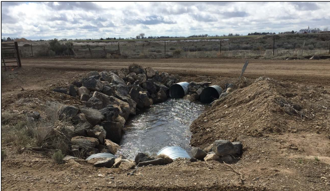
Figure 6. Culverts to Simplot Pit at Mashburn Road
