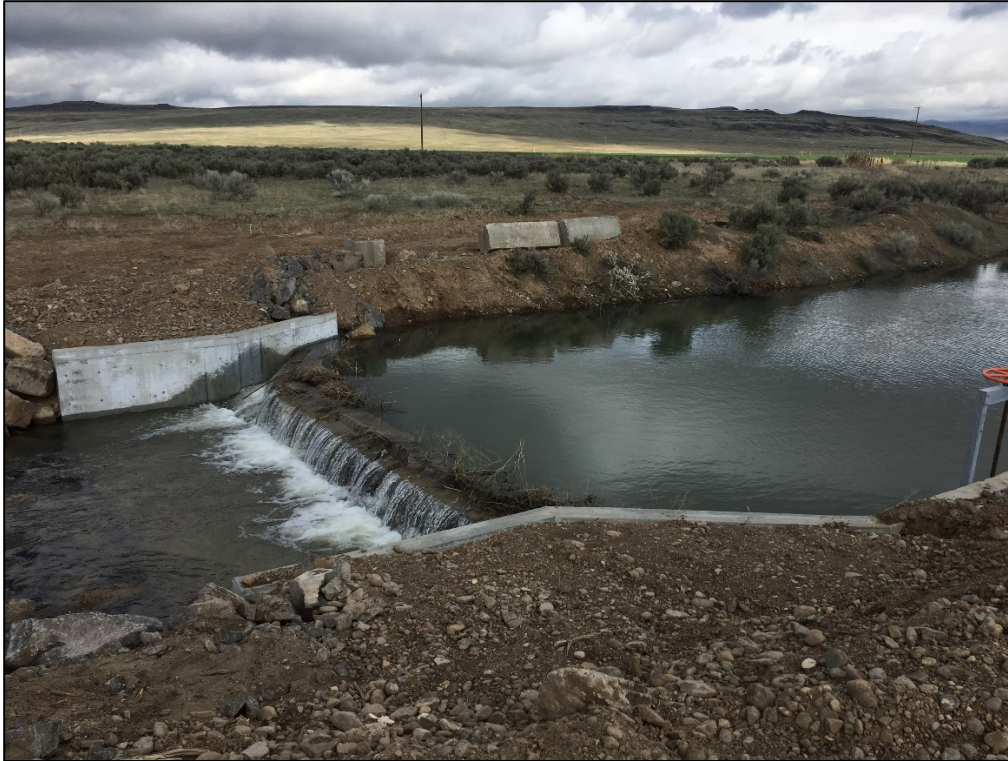
Figure 3. Check structure on Canyon Creek at BLM Pit. Removable ecology blocks are placed on concrete sill to raise the water level at the headgates.
