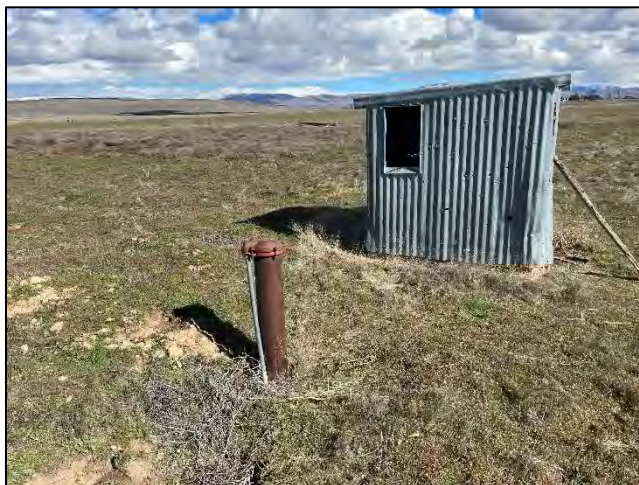
Photo 6. Pump house and clean out for on-site well.
