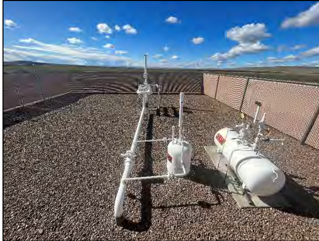
Photo 13. Natural gas tie-in for the power plant on the eastern portion of the subject property.
